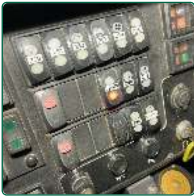
Switches and Relays
