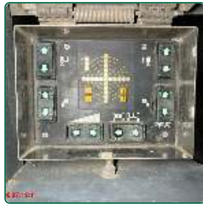
Outrigger Controls and Labeling
