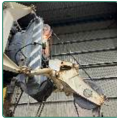
Boom Hazard Striping
