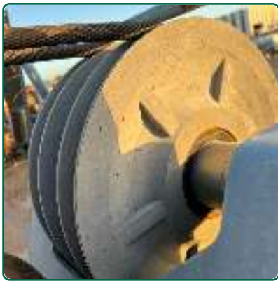
Idler Sheave and Bearing
