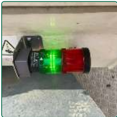
Overload Warning Lights and Alarms
