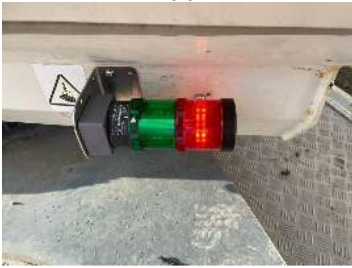
Overload Warning Lights and Alarms
