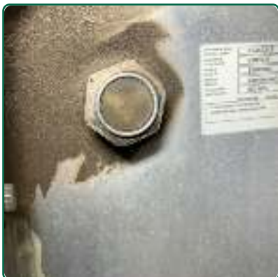
Hydraulic Reservoir & Oil Level
