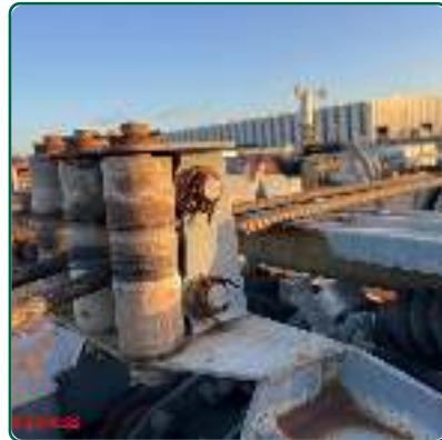
Idler Sheave and Bearing
