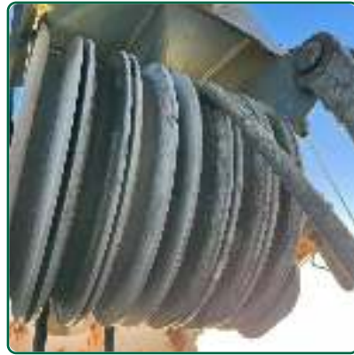
Head Sheaves and bearings
